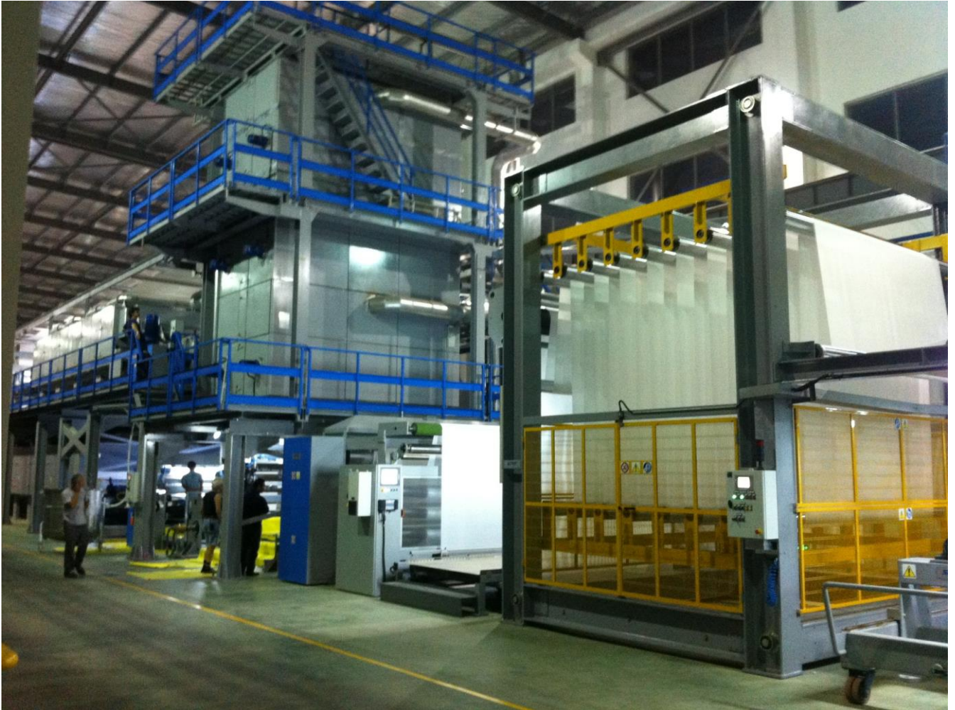
VERTICAL COATING DOUBLE SIDE + VERTICAL OVEN
