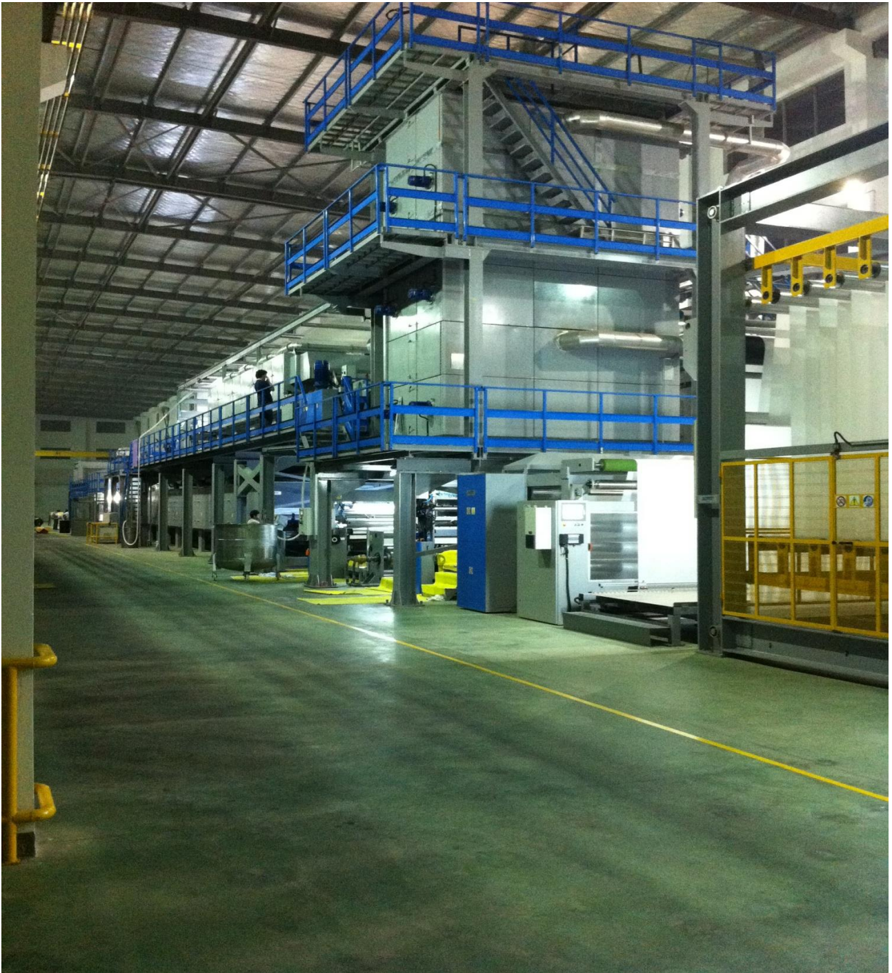
COATING LINE WITH TWO HORIZONTAL COATING HEADS
